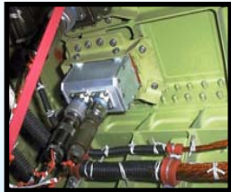
Aft Compartment Hydrogen Monitoring
