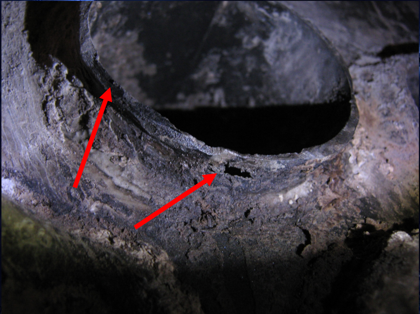
Fig.(2) : Corroded fire tube with full deterioration in the material as shown in the red arrows
