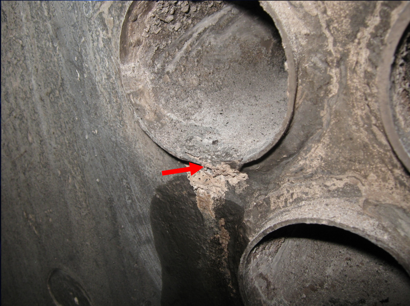
Fig.(10) : Reduction in thickness in the lower part of the fire tube with complete deterioration in the material as shown in the red arrow.
