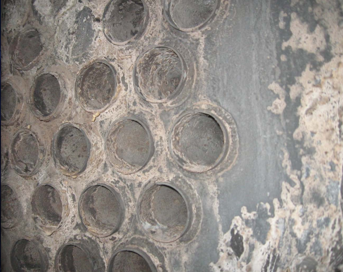
Fig.(1) : Fire tubes of the boilers
