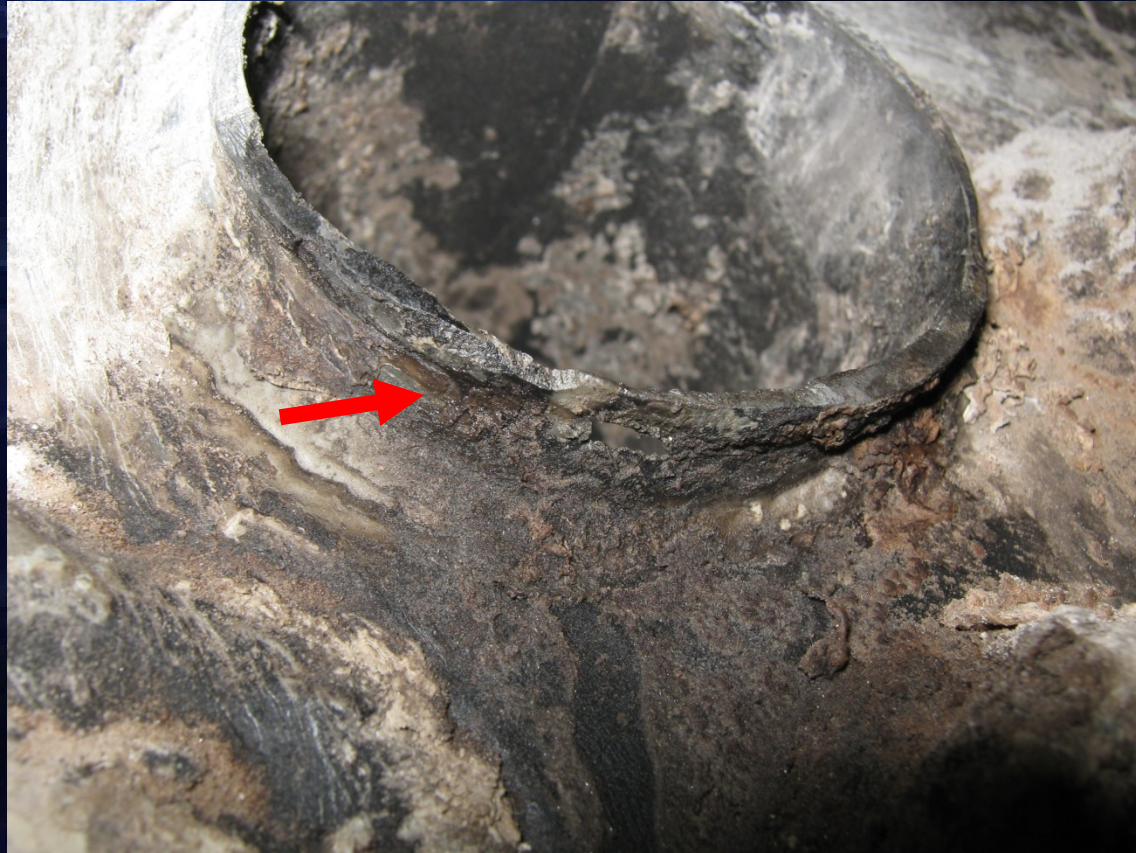
Fig.(9) : Reduction in thickness in the lower part of the fire tube as shown in the red arrow
