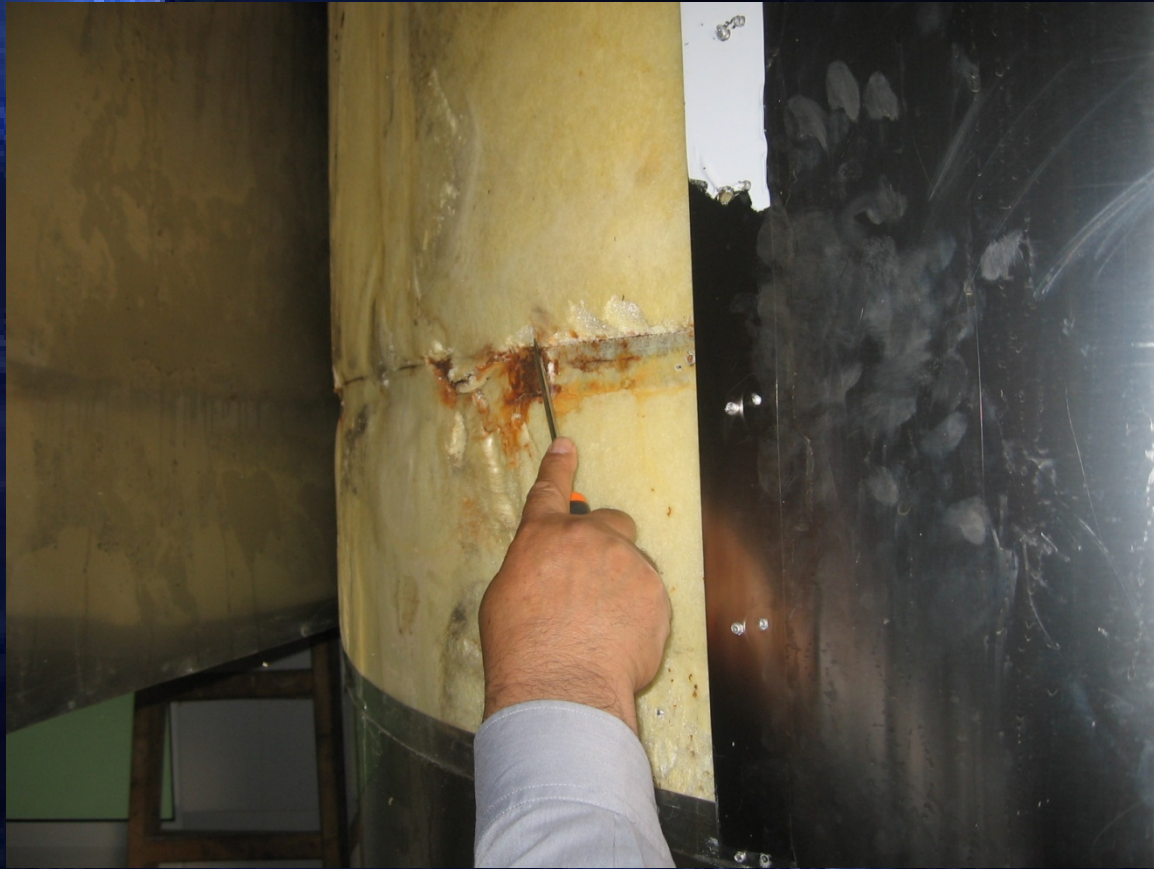
Fig.(2) : Corrosion products are very obvious below the external surface of the stainless steel sheets which appeared in the four above mentioned tanks.
