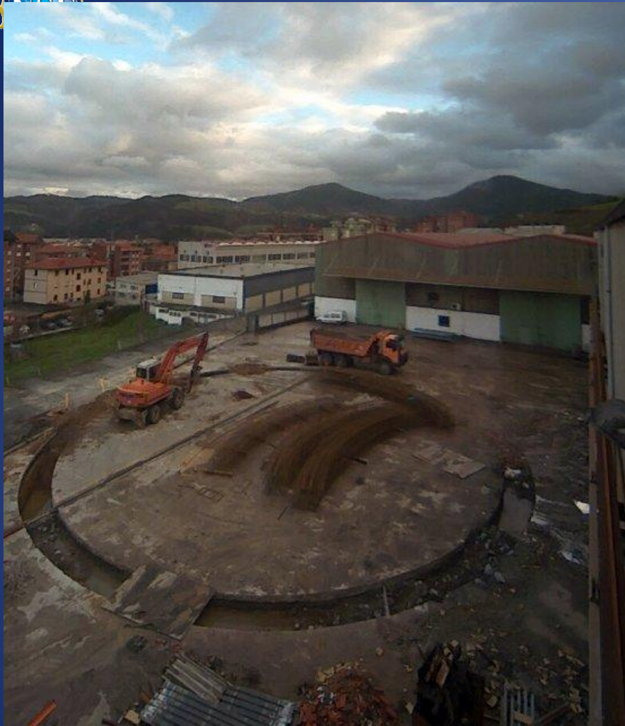
Foundation preparation for the enclosure factory assembly work in the Tallares Hilfa factory in Basauri, Spain. Image courtesy of AEC-Idom, January 2013.
