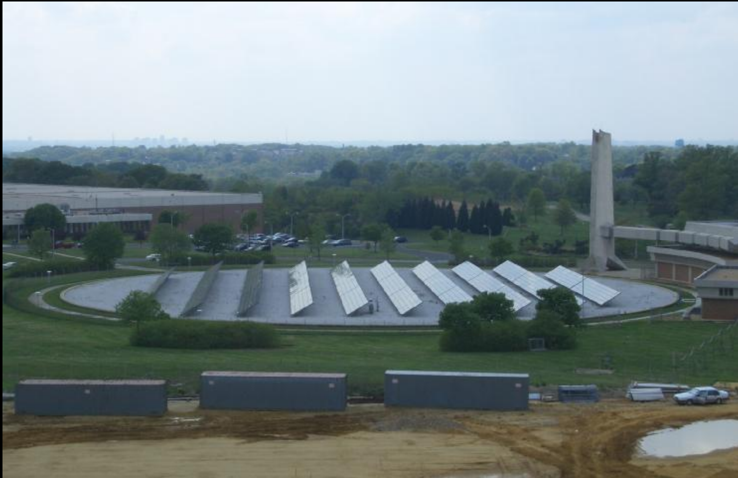
Photovoltaic Farm – Suitland, MD
