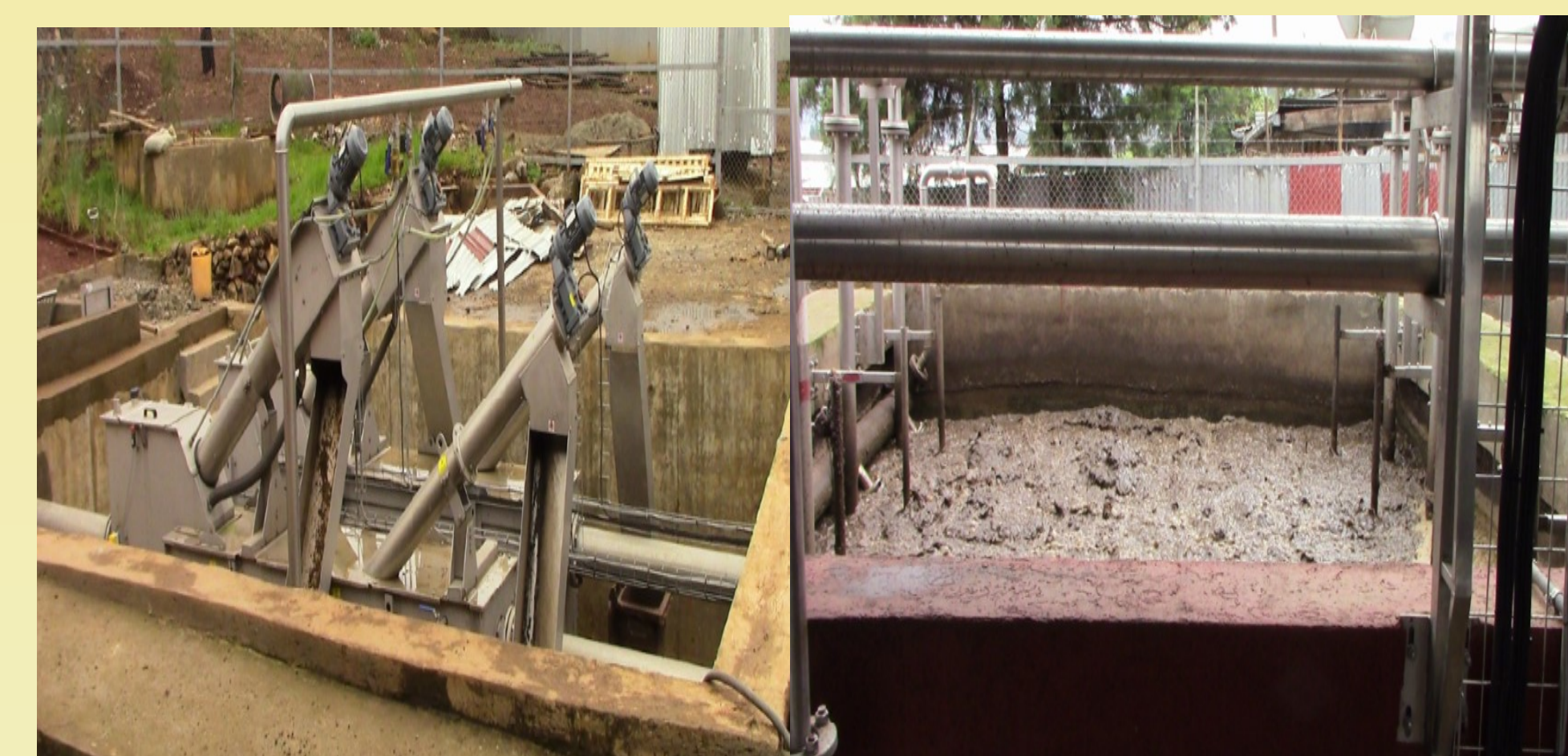
The MBR system - primary screening (left) and pre-aeration (right)
